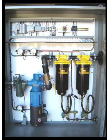
Up to 20,000 Gallon Tank
